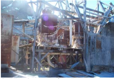
Building damage at Grytviken
